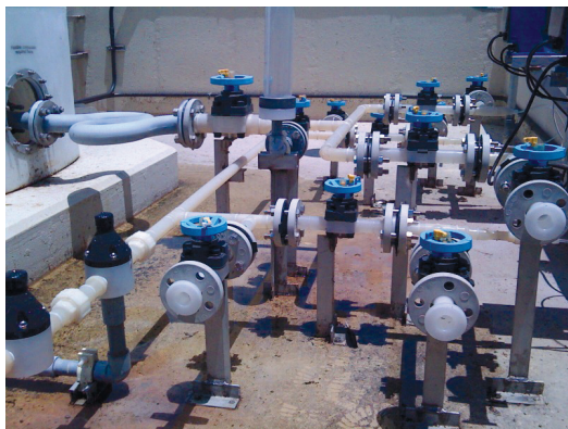
Asahi/America's Ultra Proline® for sulfuric acid distribution with T342 diaphragm valves.
