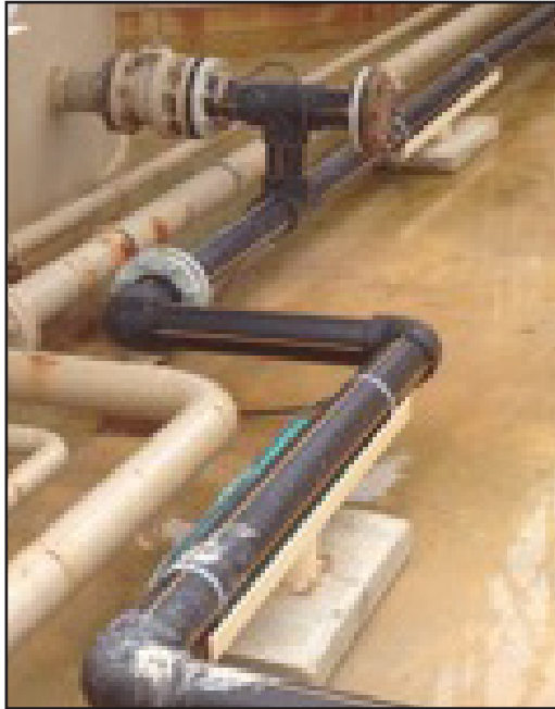
HYDROFRACTURING WATER STORAGE PLANT
